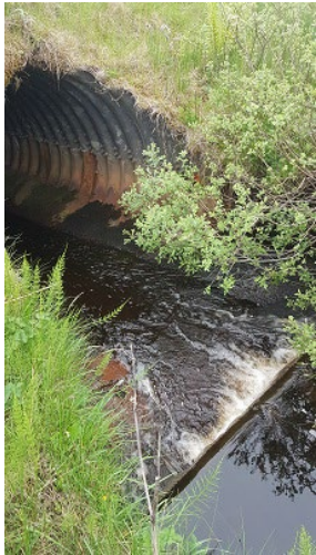
Fig. 3.1.2.5 Impassable obstacle KB03-01 (dam at upstream end of track culvert)
